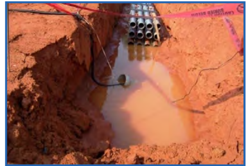
Figure 6b Water Accumulation
